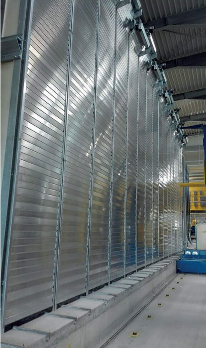
The entire system, including rack system, insulation and roller doors, was supplied and assembled by CureTec
